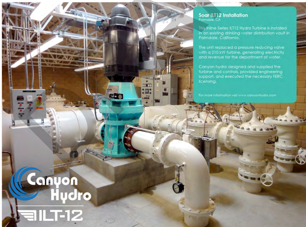
Figure 6-1: Example Hydroelectric Generation Station
